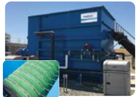
Linda County Water District, Olivehurst, CA
